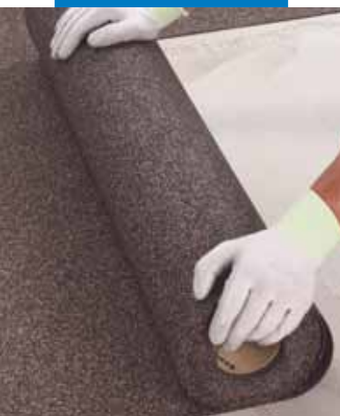
Unroll the sheets of Mapesonic CR on the surfaces to be soundproofed
