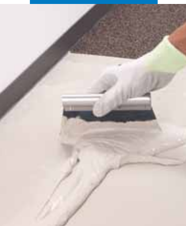
After suitable preparation of the substrate, spread on the adhesive to bond the soundproofing sheets
