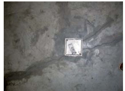
Random cracks and visual imperfection are things of the past.
