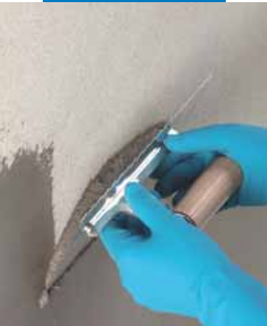
Spreading grey Fix & Grout Brick to a feather edge on the substrate
