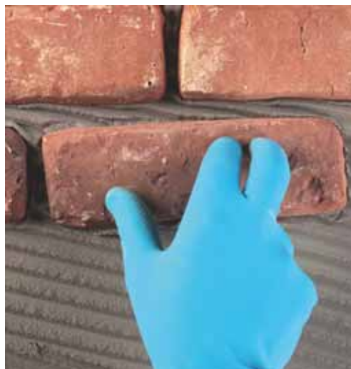
Pressing down the lath to guarantee good buttering and filling of the joints
